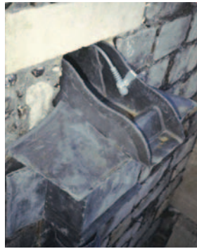
Example of a gutter sensor installation
