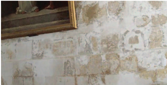
A typical example of internal wall deterioration due to damp penetration putting contents at risk
